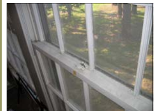
Lead dust created by the friction of opening and closing windows that have lead paint on them, is a common lead hazard.
